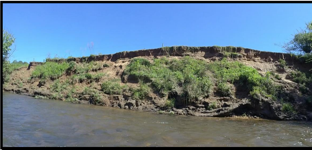
Figure 24: Example images of worst area on right bank of the Tallapoosa River between river mile 16.3 and 16.9.
