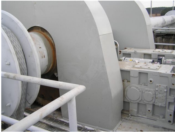
Figure 2-7. New Spillway Machinery
