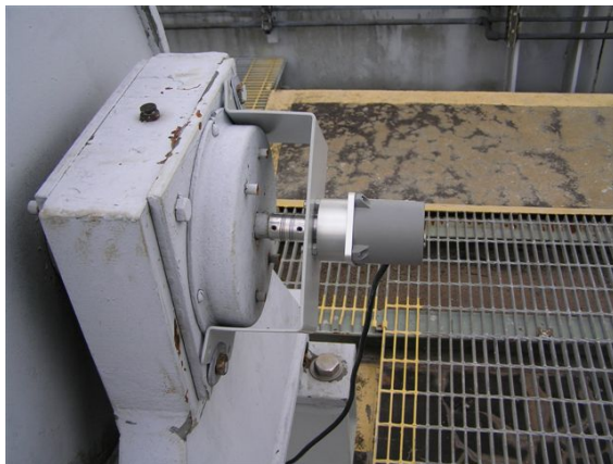
Figure 2-9. New Spillway Machinery
