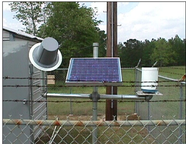
Figure 5-2. Typical Field Installation of a Precipitation Gage
