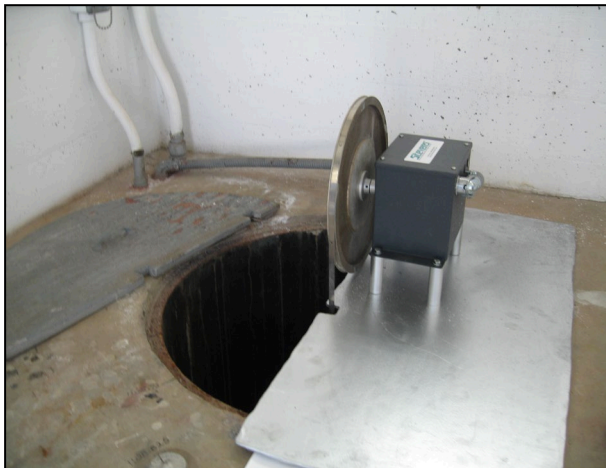
Figure 5-1. Encoder with Wheel Tape for Measuring the River Stage or Lake Elevation in the Stilling Well
