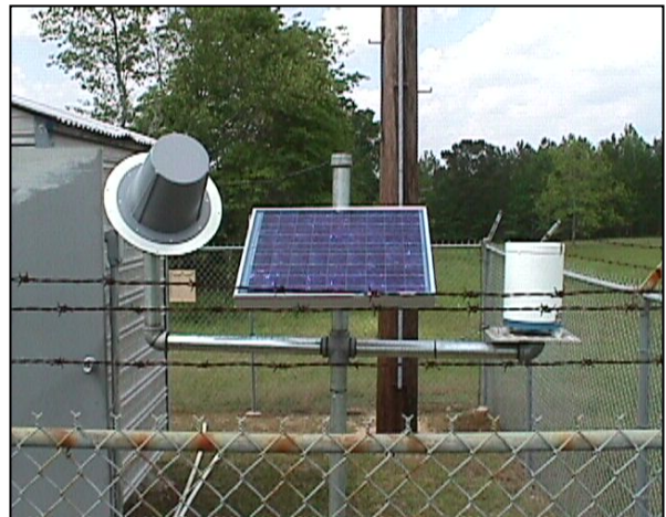
Figure 5-2. Typical Field Installation of a Precipitation Gage
