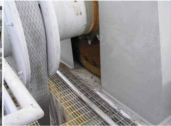
Figure 2-8. New Spillway Machinery
