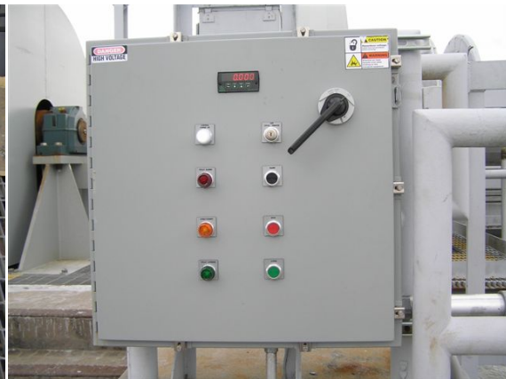
Figure 2-10. New Spillway Machinery
