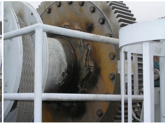
Figure 2-6. New Spillway Machinery
